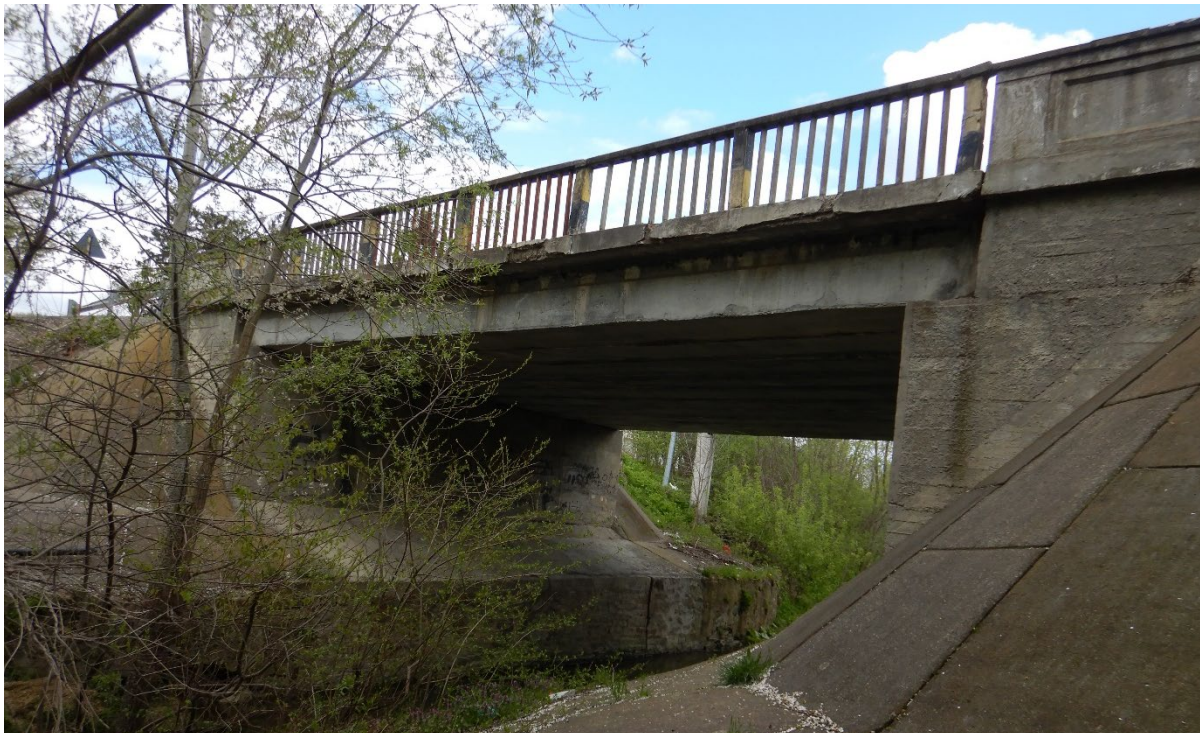
Foto 1. Vedere elevatie pod – infiltratii in grinda marginala, beton exfoliat in lisa parapet, parapet pietonal degradat
