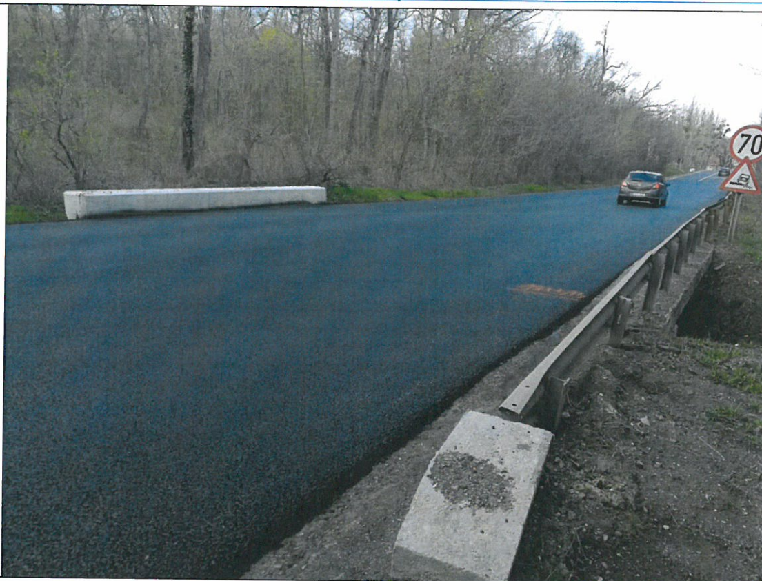
Drumul National DN 28, km 18+416 – podet transversal; parapet metalic usor deplasat spre exterior
