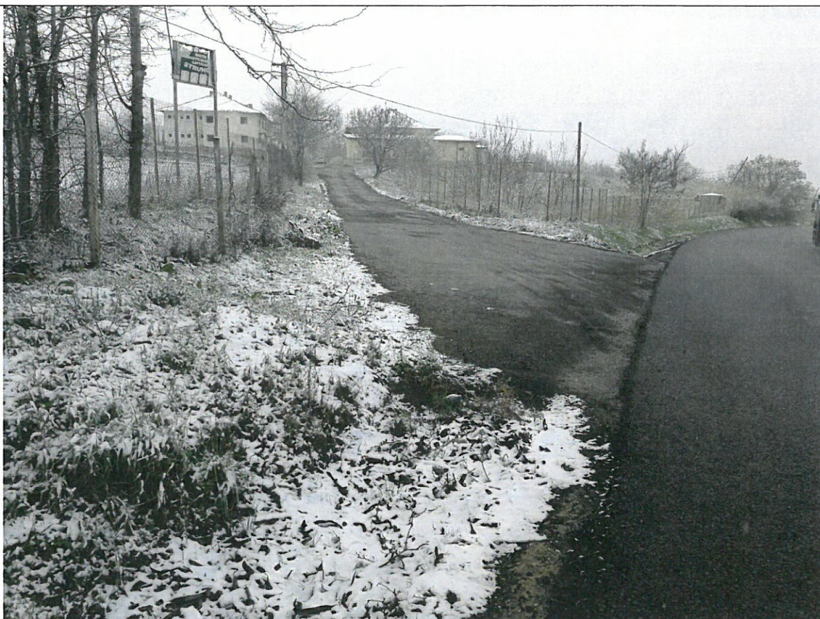
Foto 5: Drumul National DN 28, km 19+880 – drum lateral stanga; podet colmatat si inierbat;
