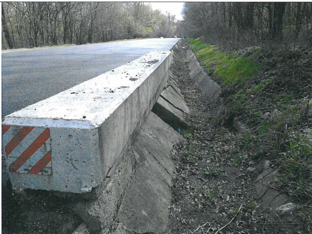
Foto 12: Drumul National DN 28, km 18+347 – podet transversal – camera de cadere colmatata in totalitate.
