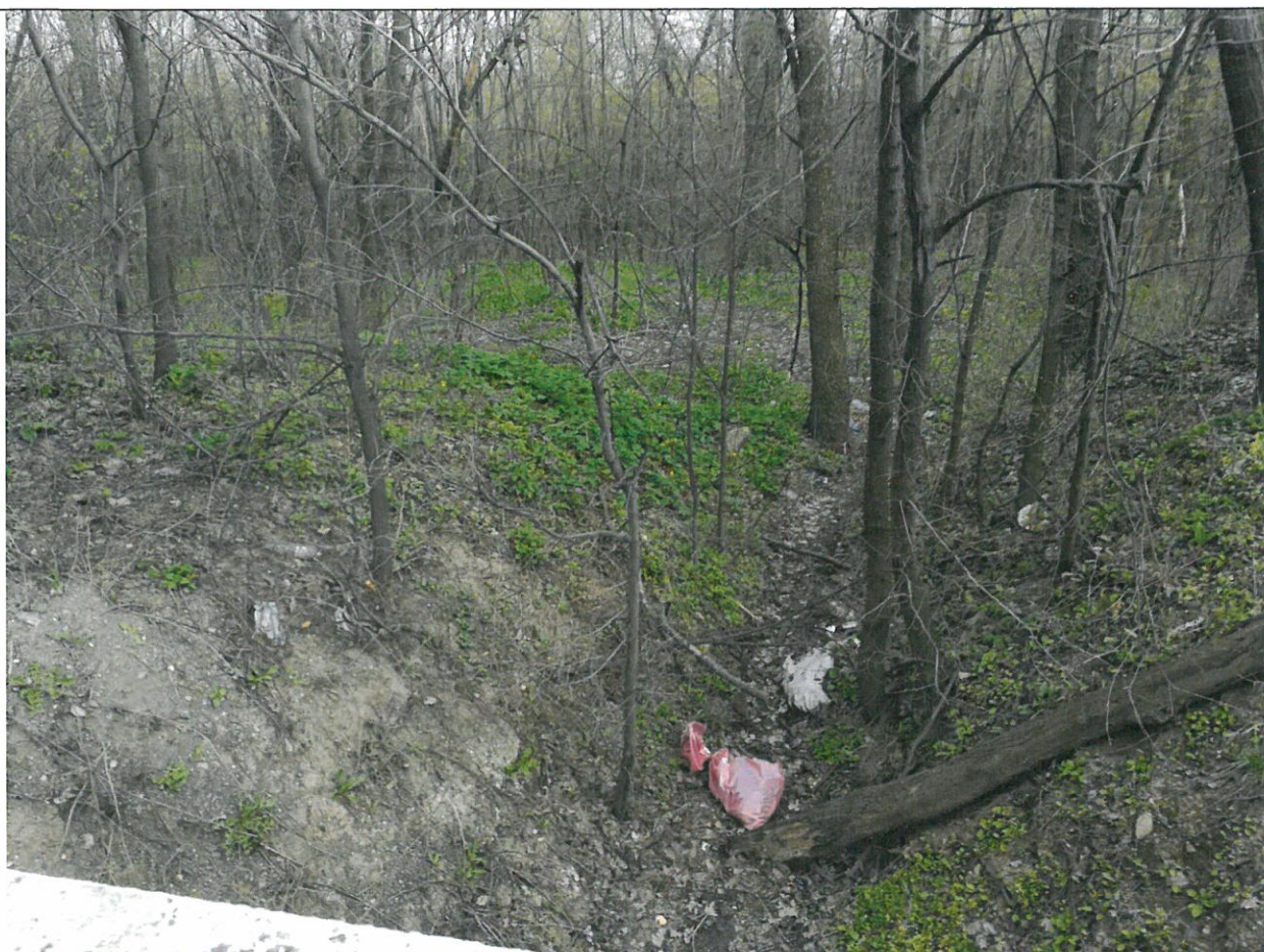
Foto 11: Drumul National DN 28, km 18+347 – podet transversal – zona aval neamenajata, vegetatie abundenta.
