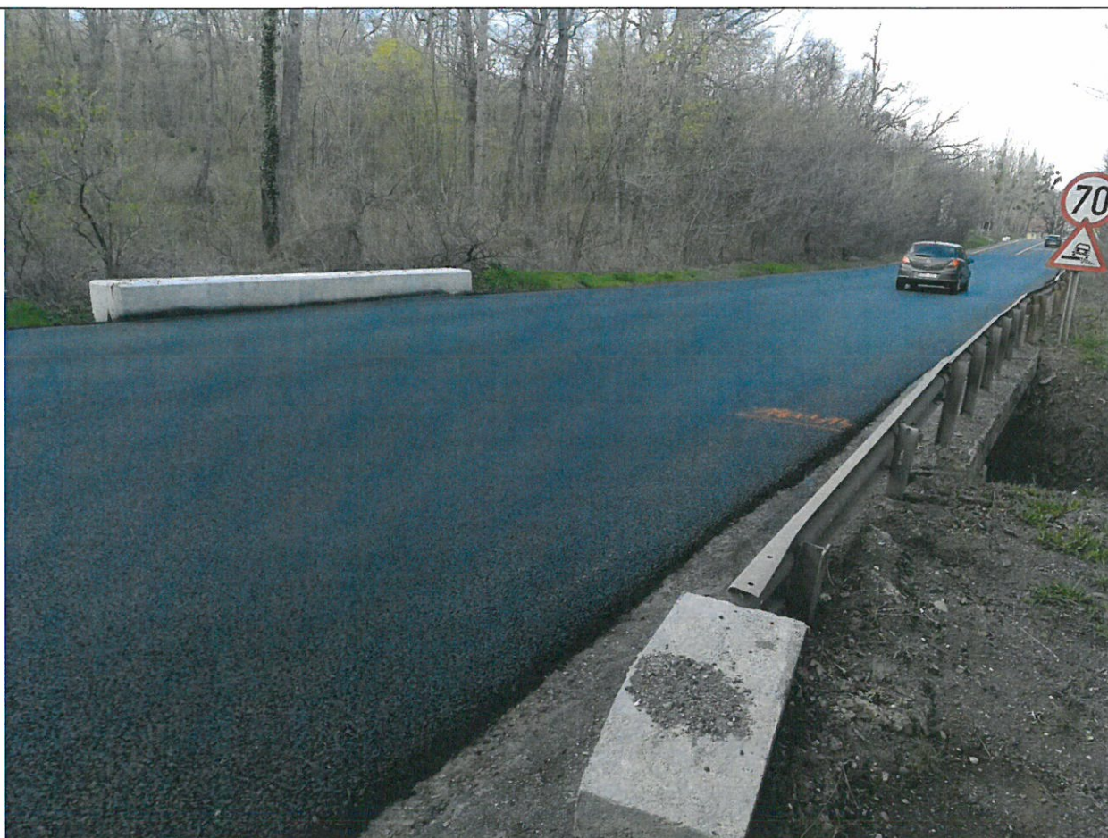
Foto 15: Drumul National DN 28, km 18+416 – podet transversal; parapet metalic usor deplasat spre exterior
