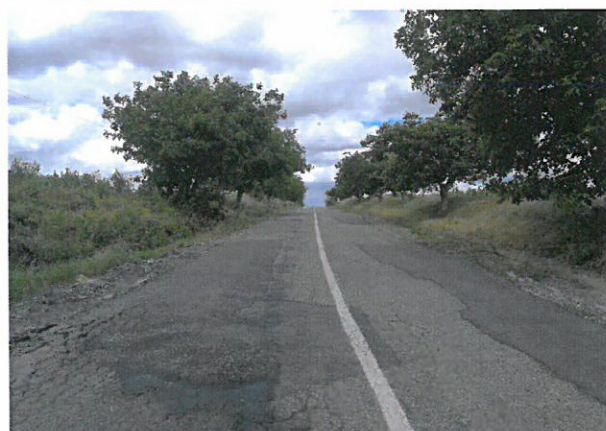
Foto 125: Drumul National DN 24C, km 105+000 – 106+000; 2 benzi de circulatie; imbracaminte asfaltica in stare rea.
