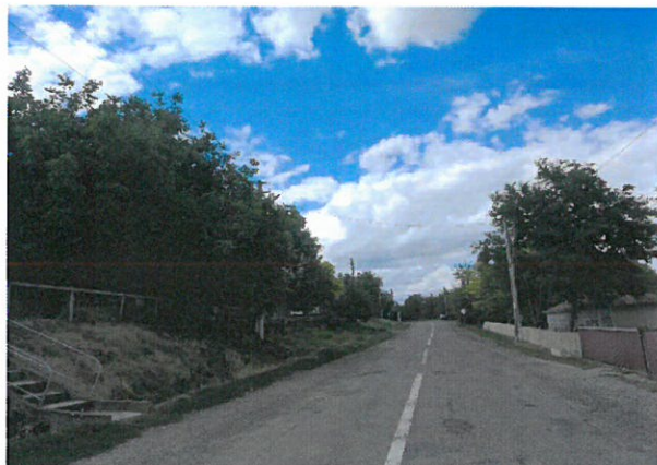
Foto 127: Drumul National DN 24C, km 106+000 – 106+663; 2 benzi de circulatie; imbracaminte asfaltica in stare rea.
