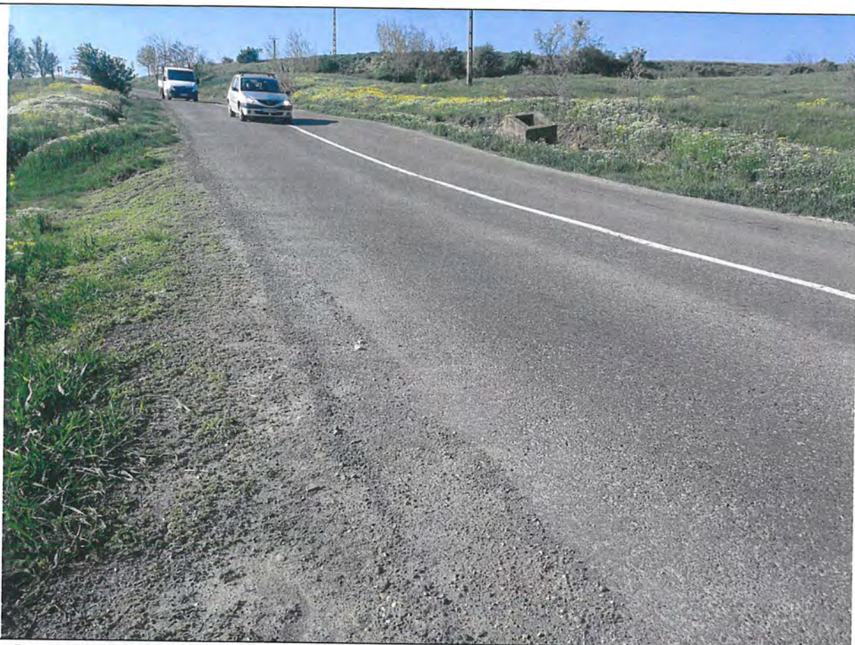
Foto 39: Drumul National DN 29, km 53+000 - 54+000 - Sector de drum national caracterizat de tasari si denivelari accentuate.
