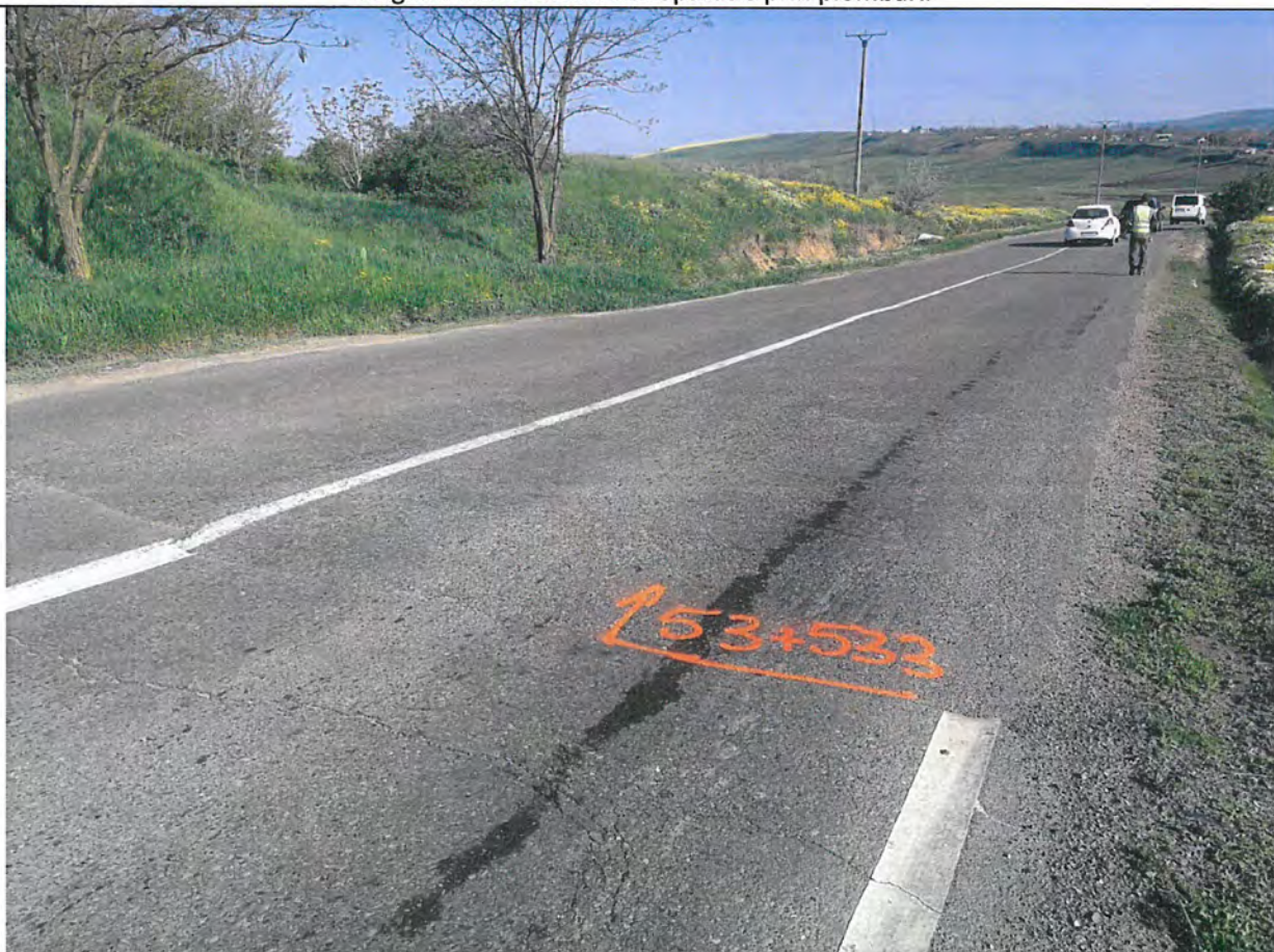
Foto 38: Drumul National DN 29, km 53+000 - 54+000 - Sector de drum national caracterizat de tasari si denivelari accentuate.
