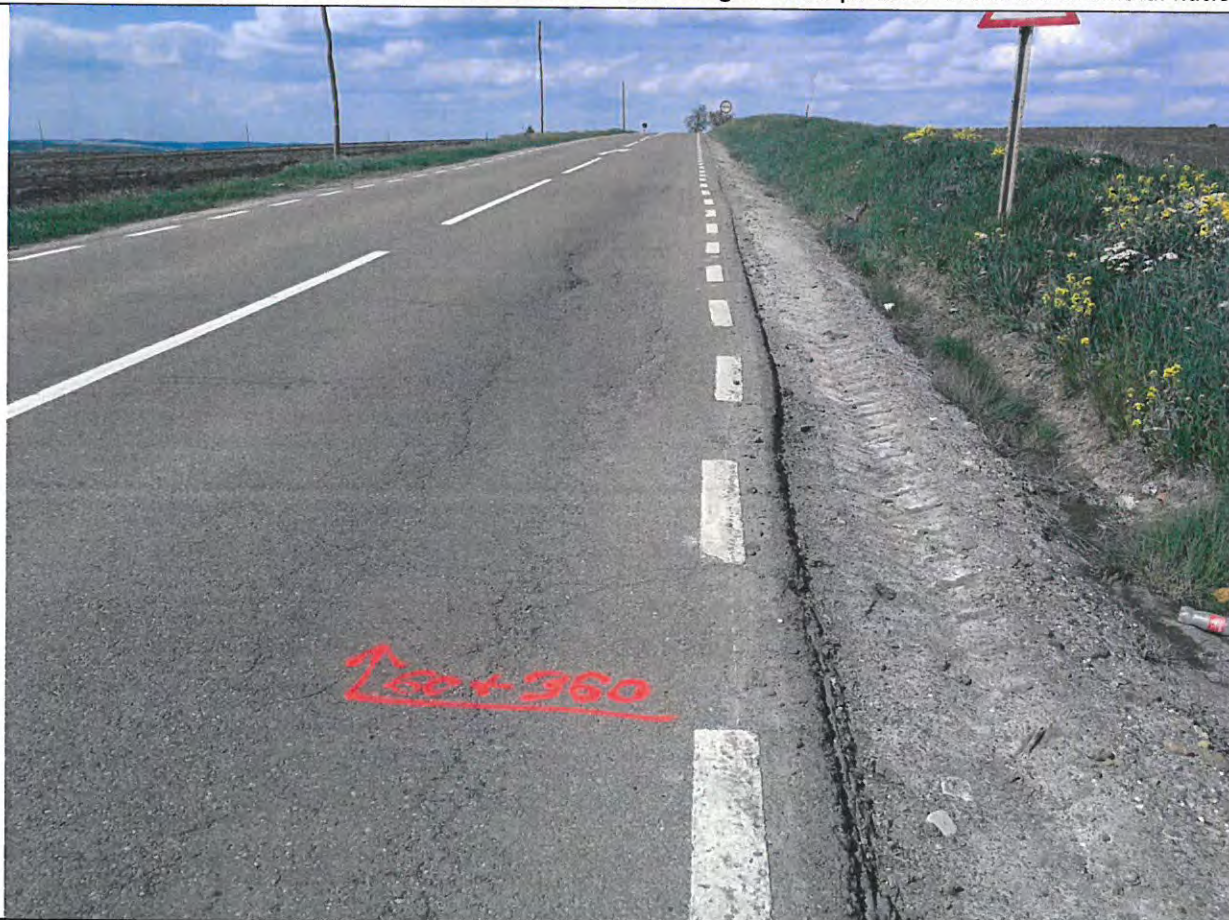
Foto 66: Drumul National DN 29, km 60+000 - 61+000 – Tasari, fagase si refulari de margine.
