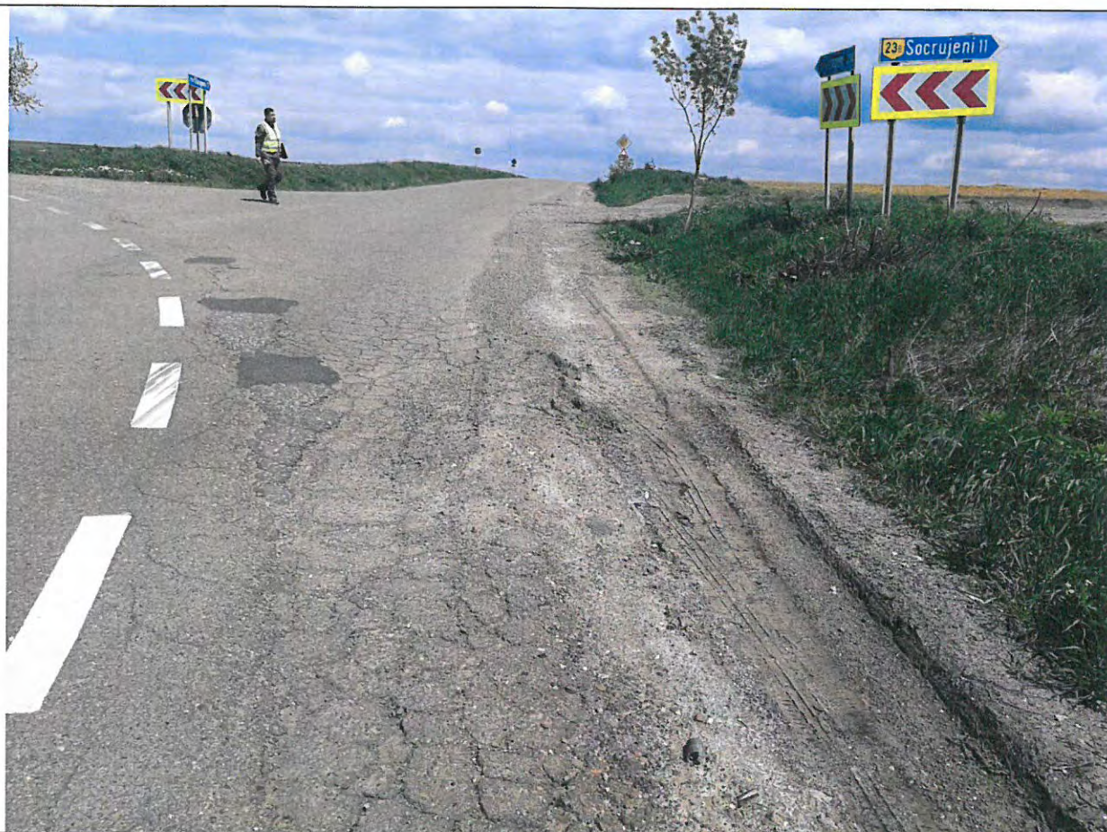
Foto 55: Drumul National DN 29, km 57+000 - 58+000 – Intersectie DN 29 – DJ 294. Acotamente distruse, Faientari pronuntate.
