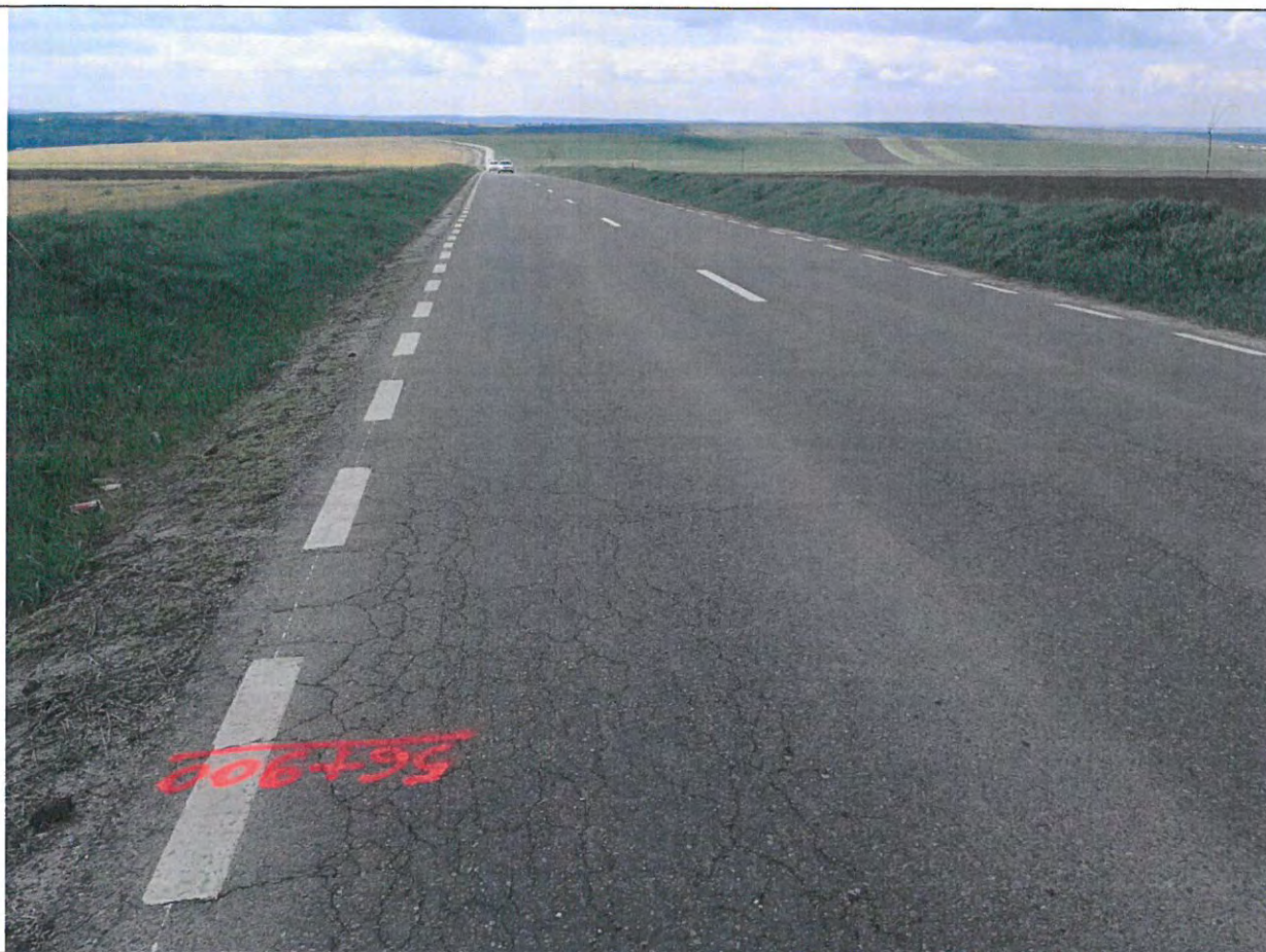
Foto 51: Drumul National DN 29, km 56+000 - 57+000 - Faientari in panza de paianjen.
