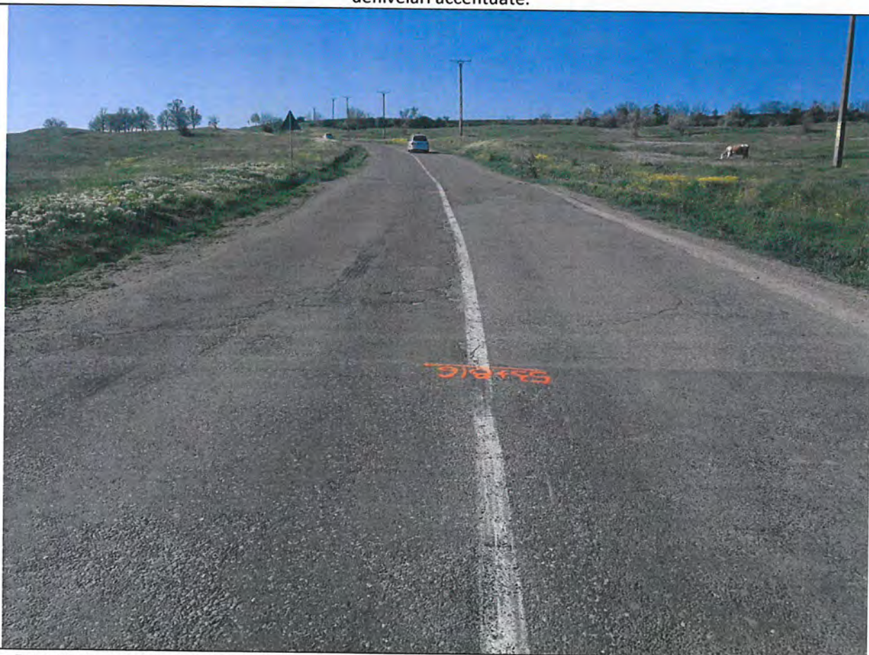
Foto 40: Drumul National DN 29, km 53+000 - 54+000 - Sector de drum national caracterizat de tasari si denivelari accentuate.
