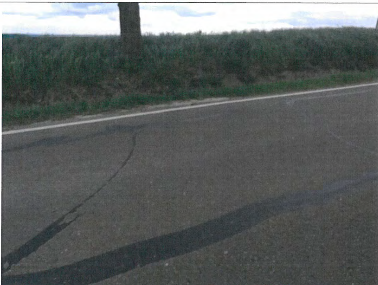
Foto 97: Drumul National DN 29, km 68+000 - 69+000 – Multiple fisuri acoperite cu mastic bituminos.
