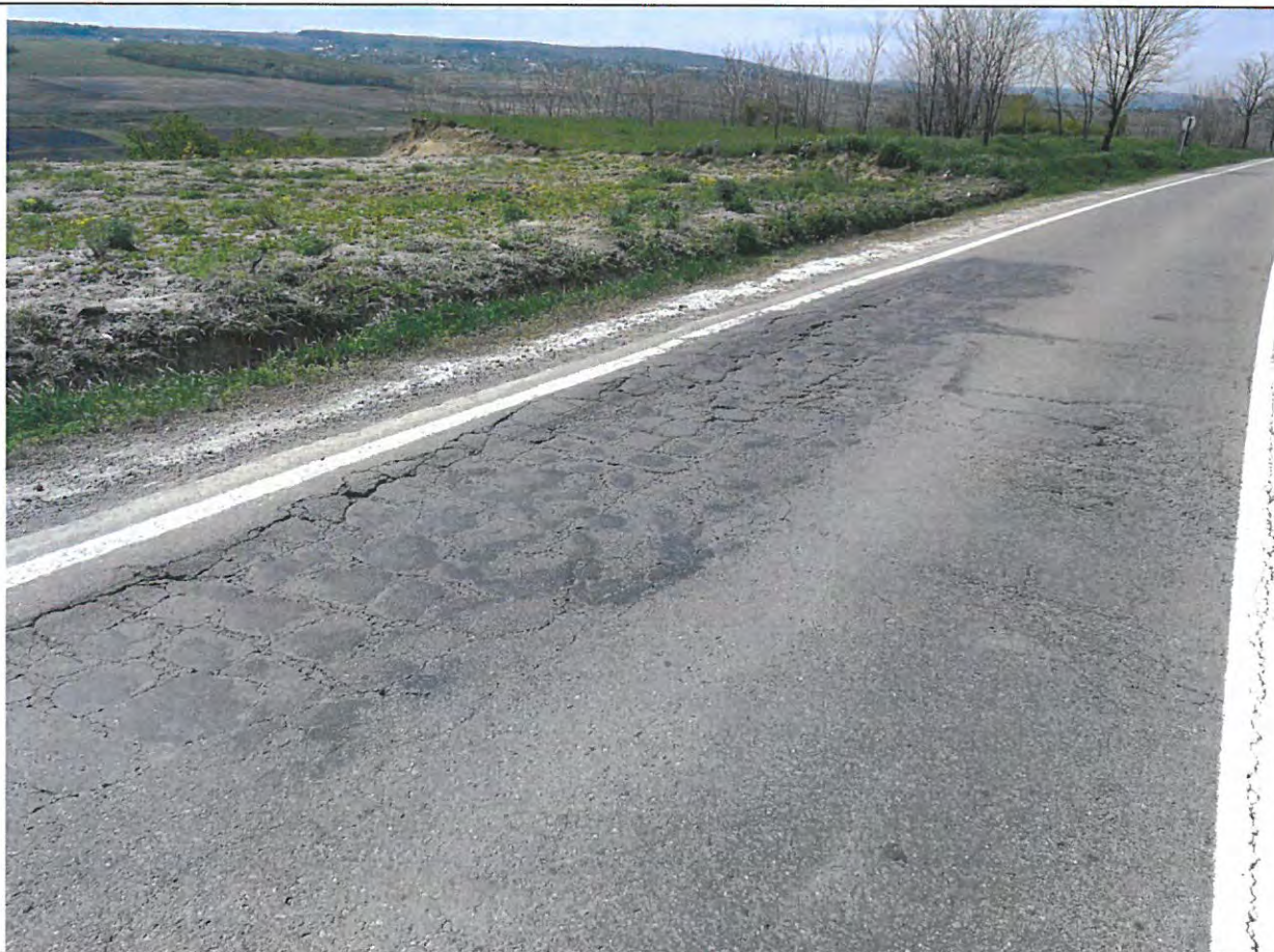
Foto 8: Drumul National DN 29B, km 7+000 -8+000 – Faientari avansate, valuriri si refulari de margine.
