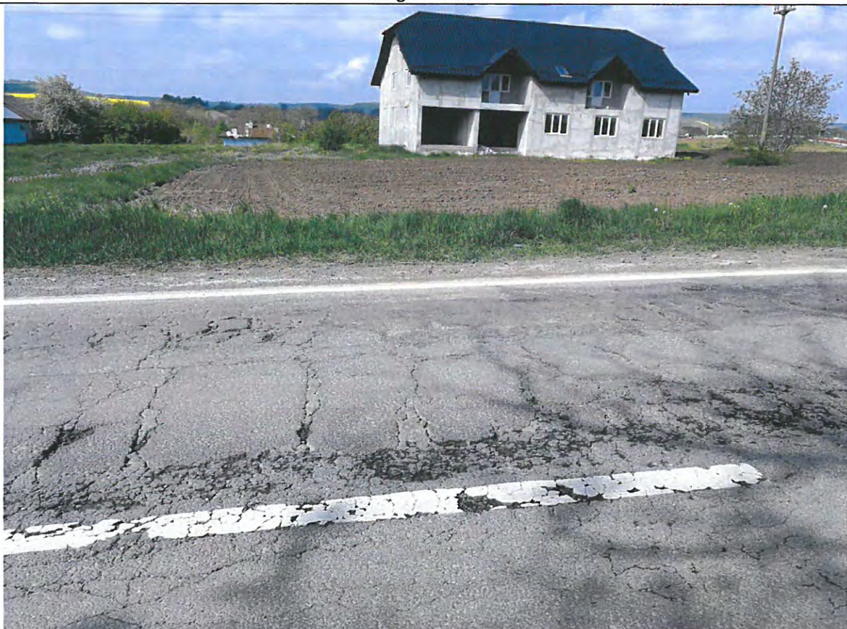
Foto 42: Drumul National DN 29B, km 16+000 -17+000 – Crapaturi transversale, fagase, faientari.
