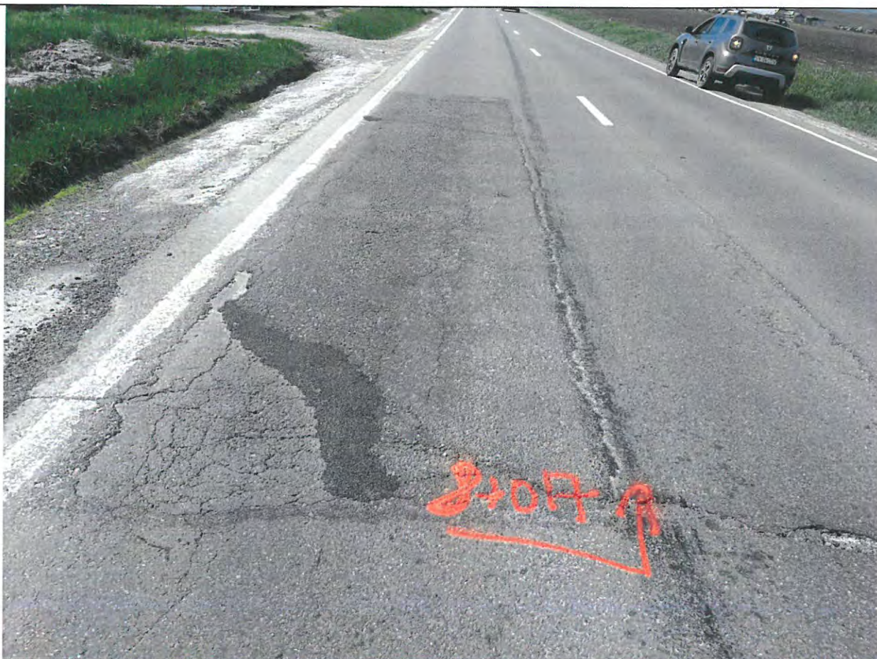
Foto 9: Drumul National DN 29B, km 8+000 -9+000 – Lucrari de reparatie locale (plombari), desprindere mixtura, faiantari in panza de paianjen.
