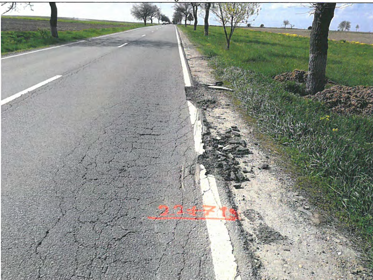
Foto 68: Drumul National DN 29B, km 22+000 -23+000 – Refulari de margine. Rupturi ale mixturii asflatice in zona acostamentelor.
