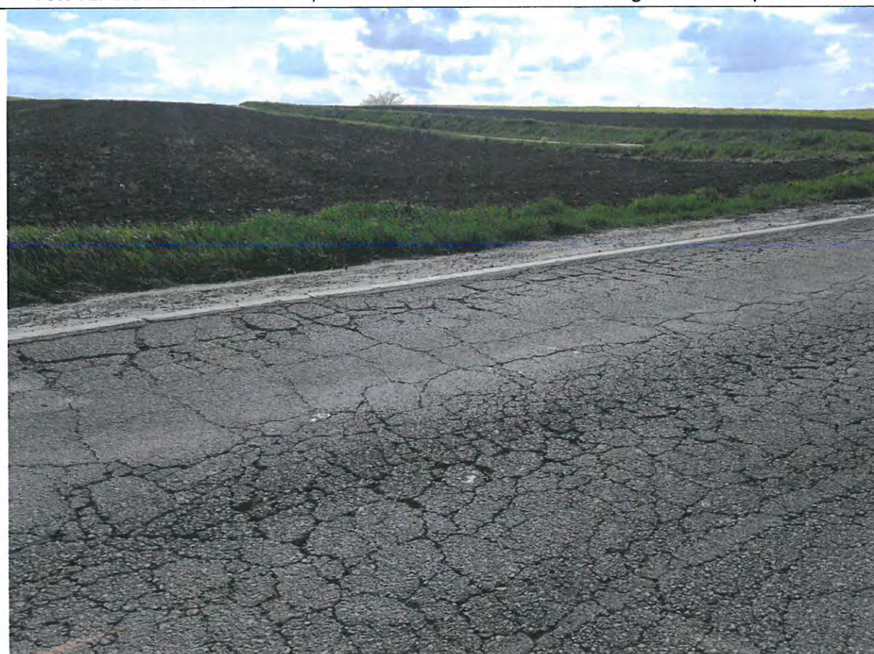
Foto 72: Drumul National DN 29B, km 23+000 -24+000 – Refulari de margine. Faiantari pronuntate.
