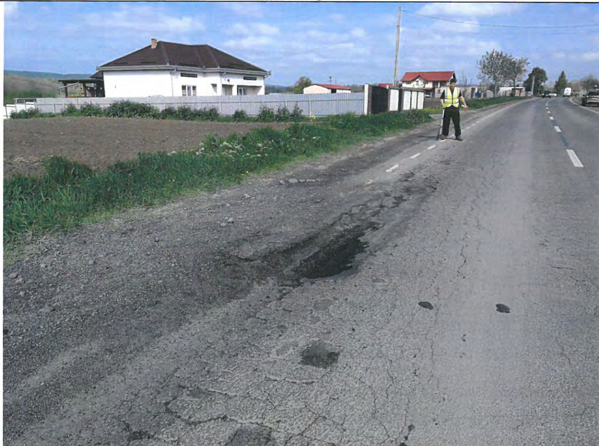
Foto 40: Drumul National DN 29B, km 15+000 -16+000 – Gropi, faientari si refulari.
