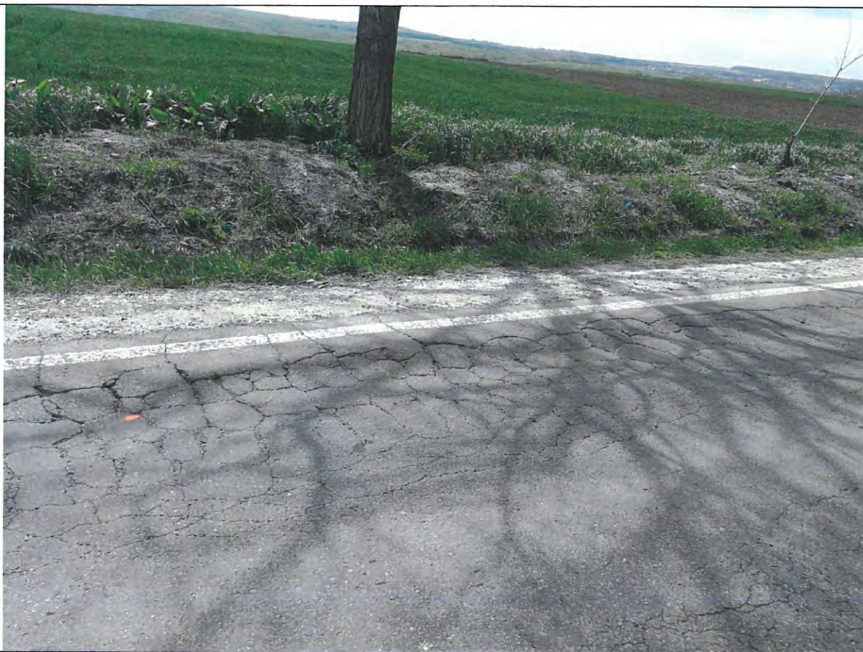
Foto 7: Drumul National DN 29B, km 7+000 -8+000 – Faientari avansate, valuriri si refulari de margine.
