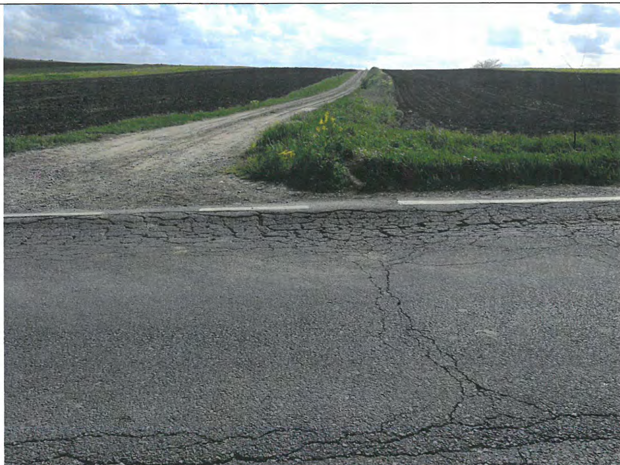
Foto 71: Drumul National DN 29B, km 23+000 -24+000 – Refulari de margine. Faiantari pronuntate.
