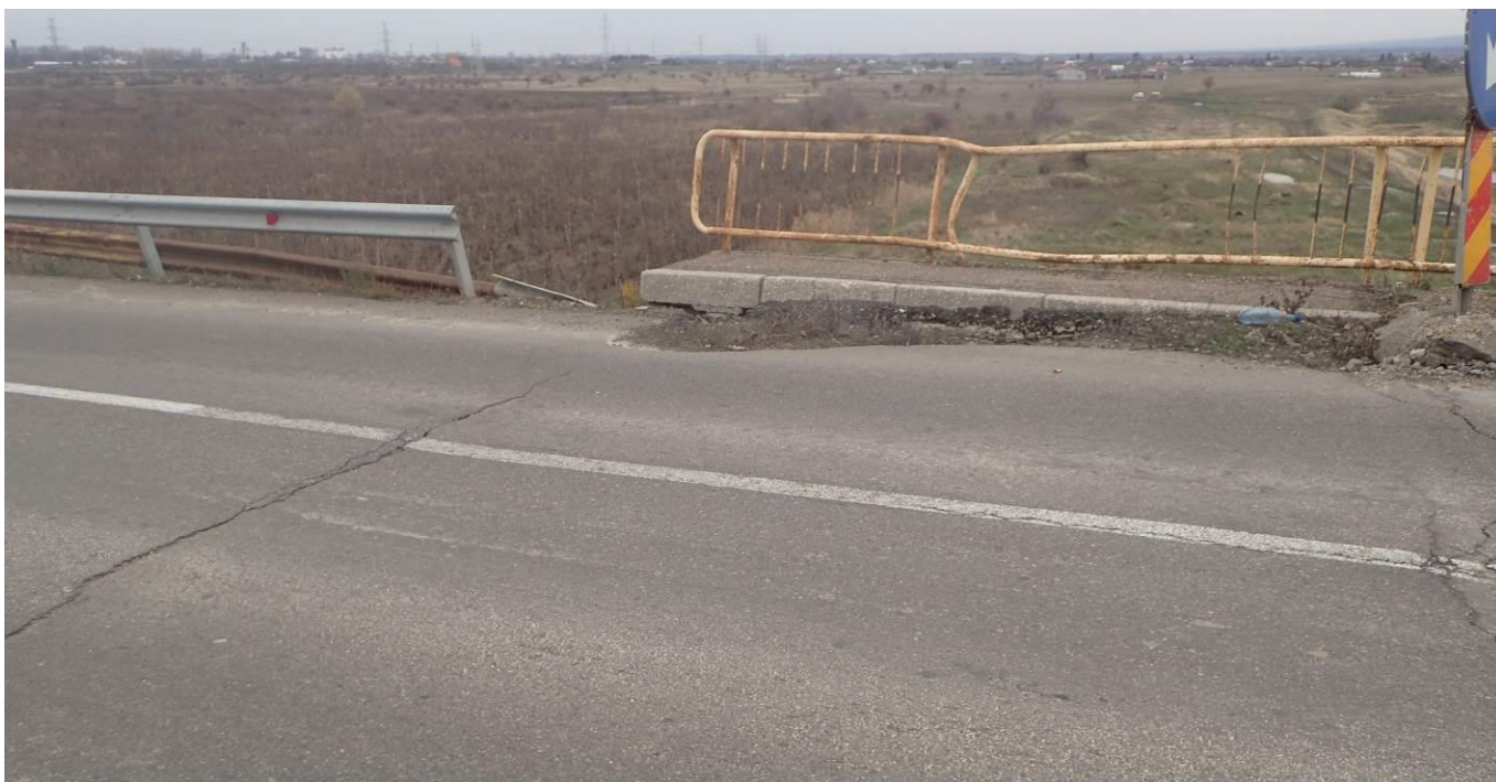
FOTO 27. Parapet deformat atat in plan orizontal cat si vertical, tasari in ale rampei in zona placilor de racordare
